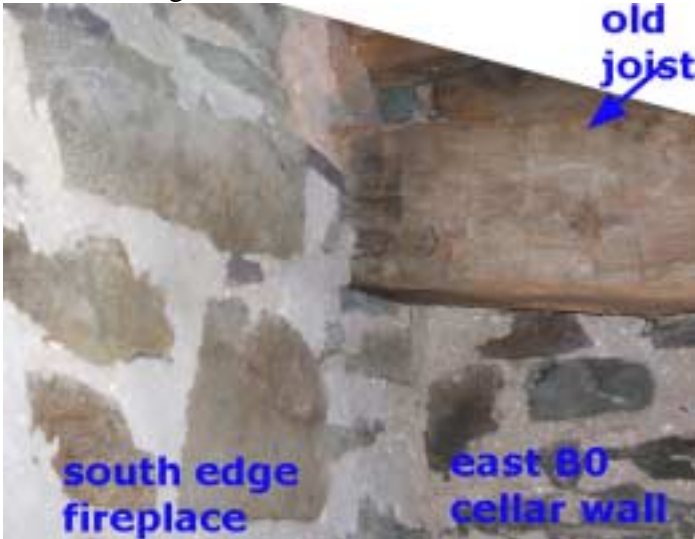
Close-up of old floor joist along east wall of "B0" embedded in south end of fireplace mass. Current floor joist directly above it.
