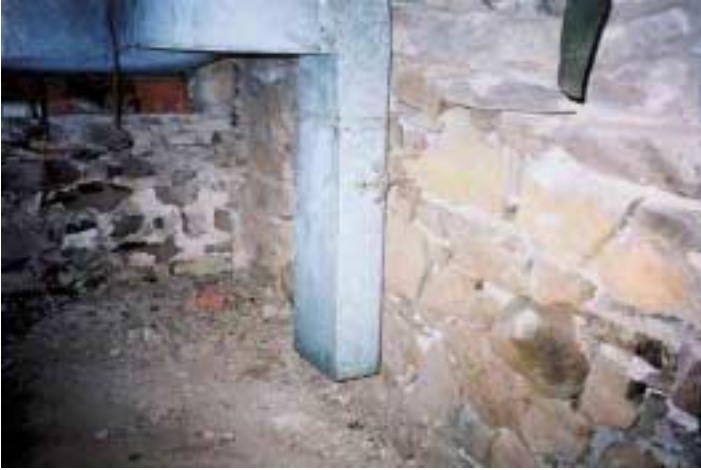
North wall & crawl-space entrance visible under duct work. Vertical duct abuts west face of "B0" fireplace mound hearth extension. Note variation in hearth extension finish.
