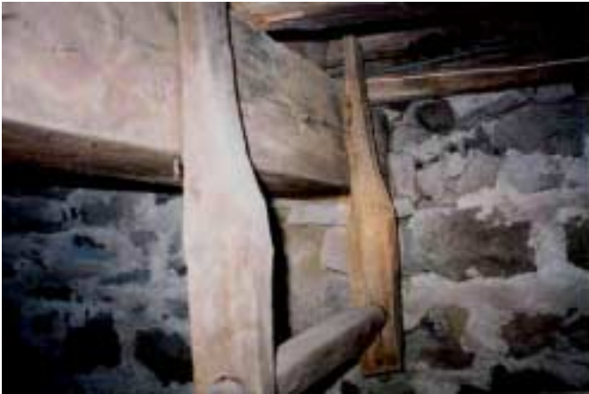
Storage rack hanging from central East-West summer beam under 1st floor joists in "B0" cellar. West end of beam rests in large pocket on west wall. (Other end is embedded in fireplace mass.)
