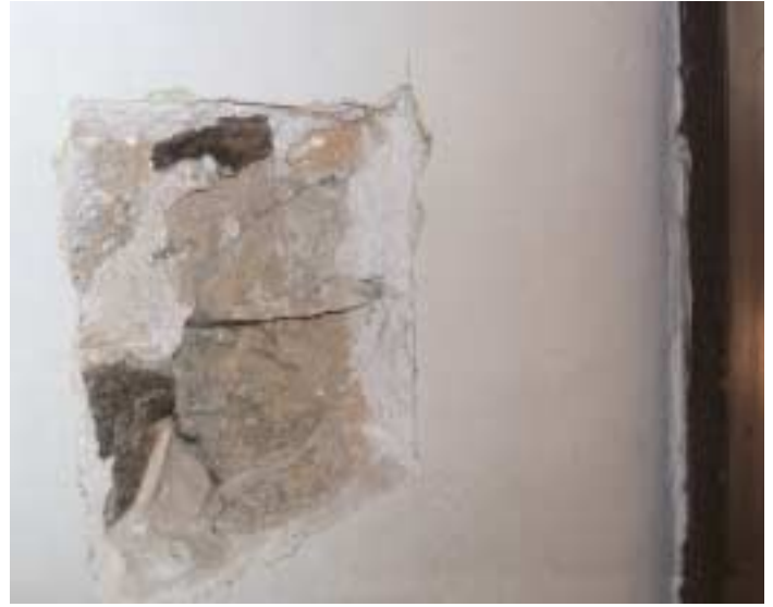
Removal of plaster to take mortar sample M13 from south side of south jamb of unit "B1" fireplace reveals fireplace construction. Door from "B1" to "C1" visible to right.
