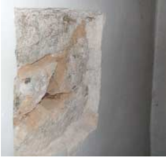
Exposed stone and mortar (M19) from north corner of west wall of room "B108", between cellar stairs and north window. This mortar contains horse hair, an older formulation than all the other samples.
