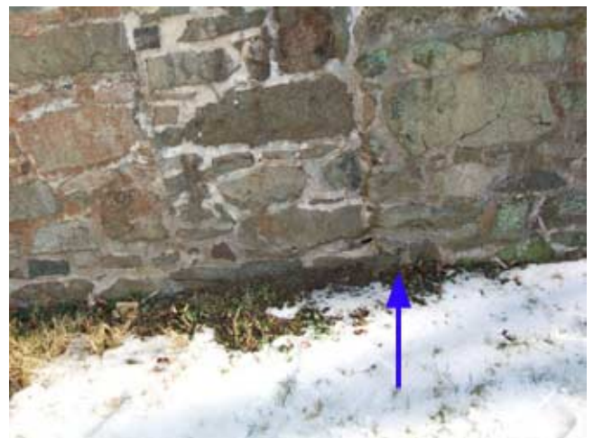
North wall Vertical seam jogs 4" to the east from unit "A", resulting in a ground-level notch
