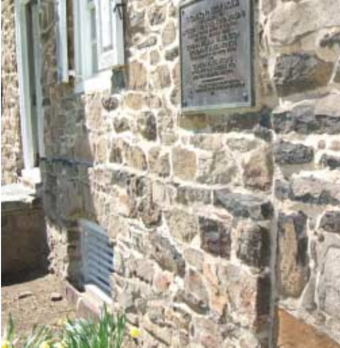
South exterior of unit "A". water table protrudes horizontally midway between cellar and 1 st floor windows. It is noticeable in jagged shadow and shadowed edge at "A" – "B" vertical mortar seam
