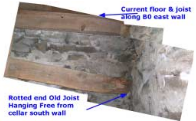
Close-up of rotted south end of old floor joist now disconnected from south "B0" cellar foundation and dangling free.
