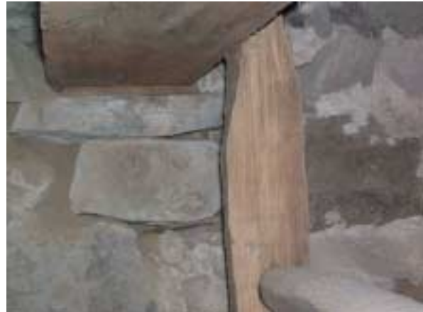
West end of summer beam rests on loosely piled rocks filling the pocket to bring the beam from its original position when unit "A" & this wall were built to its new position when hearth extension built..
